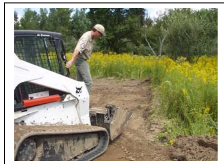
Jeremy Shafer checks over the ephemeral pool construction at the Homer Lake wetland complex area.
